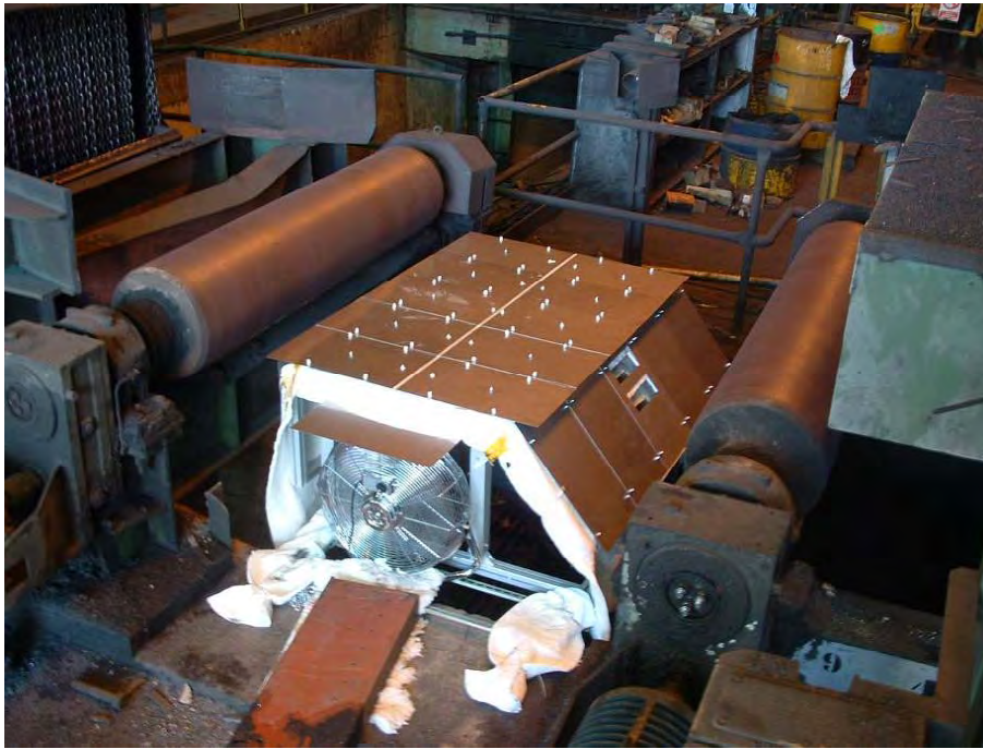
Fig. A2.9: Plant installation at Arcelor for bottom face crack inspection The structure with the sensor is placed underneath the strand, with a thermally insulated shield on top of it and a fan to provide fast moving, cool air
