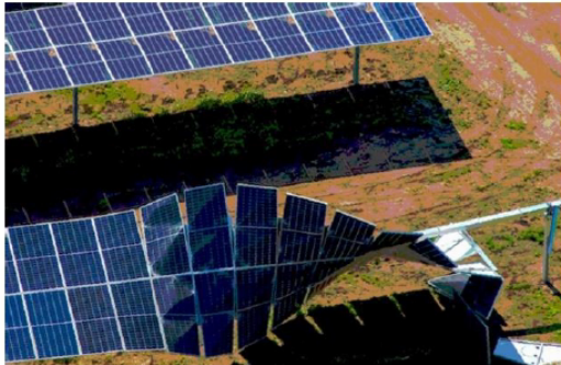
Fig. 2 Collapse of a single-axis solar tracker facility (rendering)
