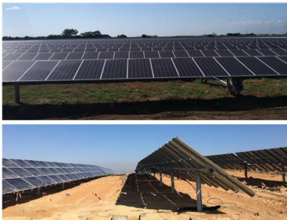
Fig. 1. Solar tracker plant.
