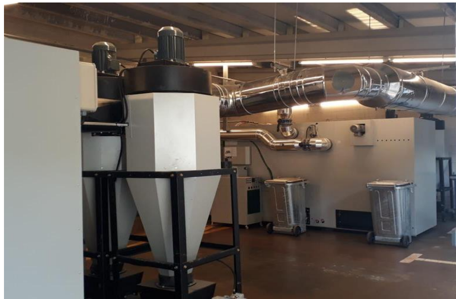
Figure 8. Thermal system in the Pontevedra campus of the University of Vigo.
