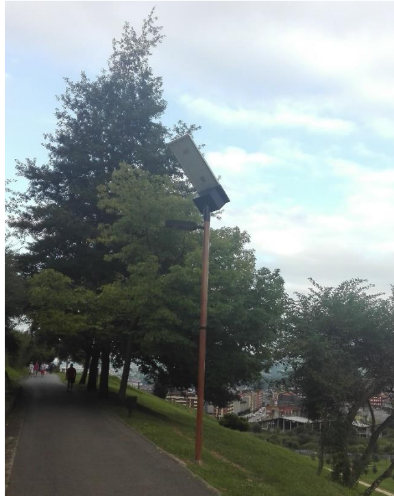
Fig. 4. Solar self-consumption system for lighting solutions.
