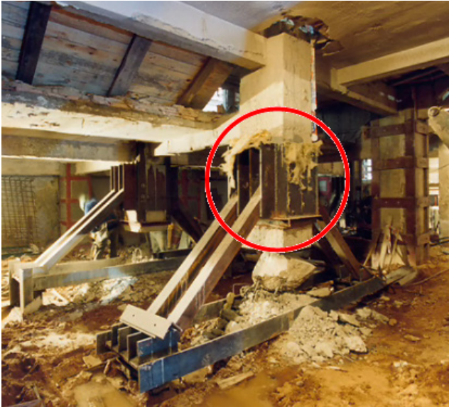
Figure 5. Joint seal between the auxiliary structure to the pillar using epoxy resin
