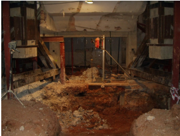
Figure 9. Demolition of the lower part of the pillars and the original footing
