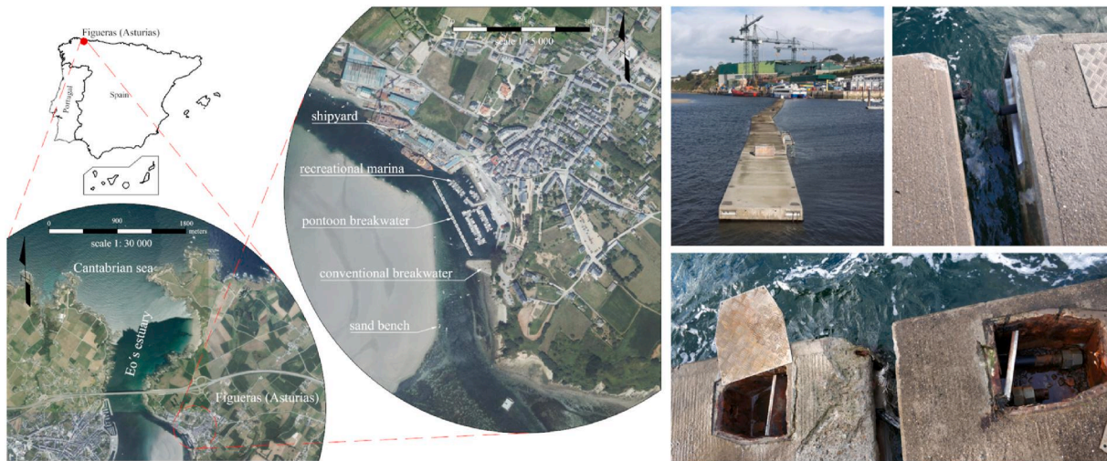
Fig. 2. Floating breakwater at the Port of Figueras (Spain): location (left) and pictures of the structure after connector breakage (right).
