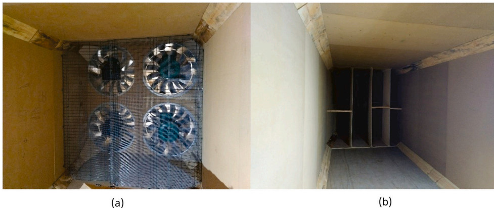
Fig. 5. View of the secondary chamber. (a) Suction of the fans. (b) Deflectors.
