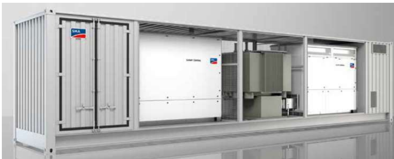
Figura 25. MV Power station 6000 de SMA[28].
