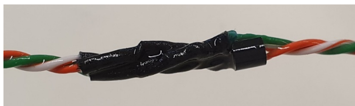
Figure 11. Sensor located on the 1-wire cable.
