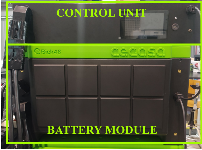
Fig. 13. Setup used for the experimental results. The battery module consists of 15 LFP cells in series.
