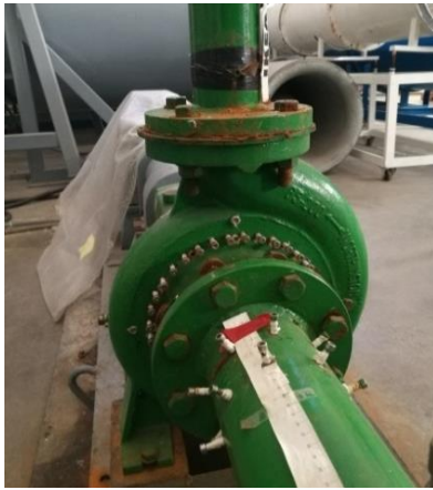
(a) Test pump
