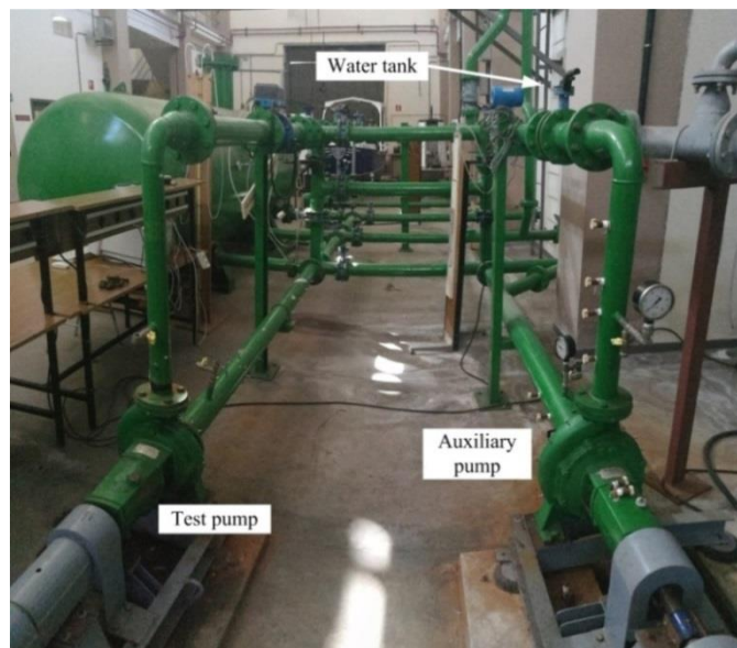
Fig. 3.4. Photograph of the hydraulic circulatory system
