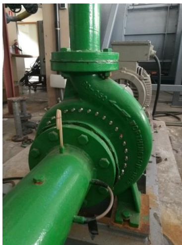
Fig. 3.1. Photograph of the auxiliary pump
