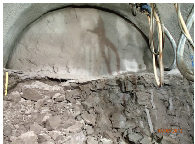
Fig. 13. Circular failure during bench stage.
