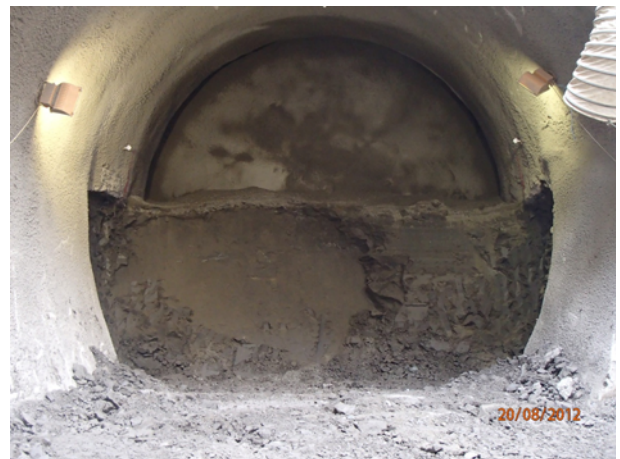
Fig. 12. Planar failure during bench stage.
