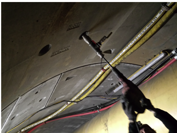
Fig. 9. Proof drilling through the grouting port of the TMB tunnel segments with handheld equipment.
