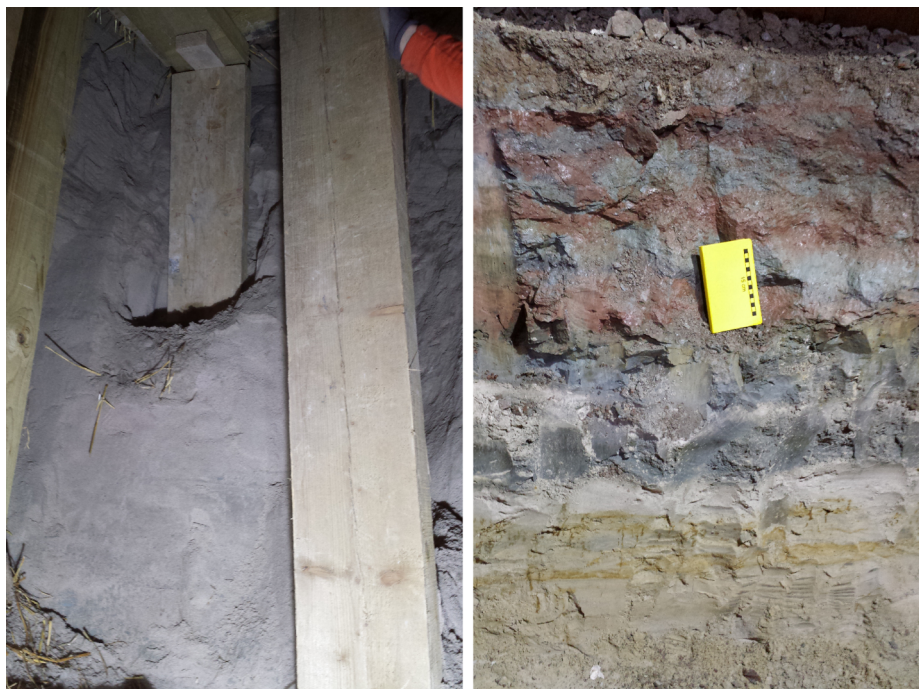
Fig. 20. View of excavation of the sand channel in the crown of the cross passage, on the left. On the right, view of boundary of the Upper Mottled Beds underlain the Laminated Beds.
