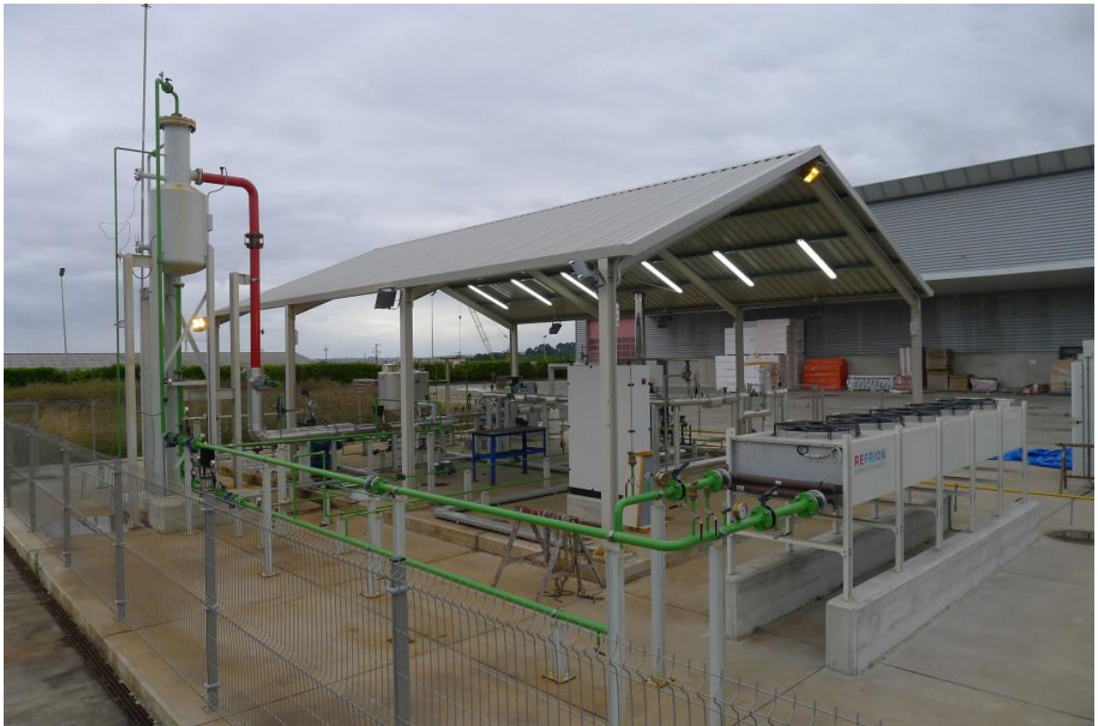
12 13 Figure 2. HCT test plant with detail of the dry coolers used.
