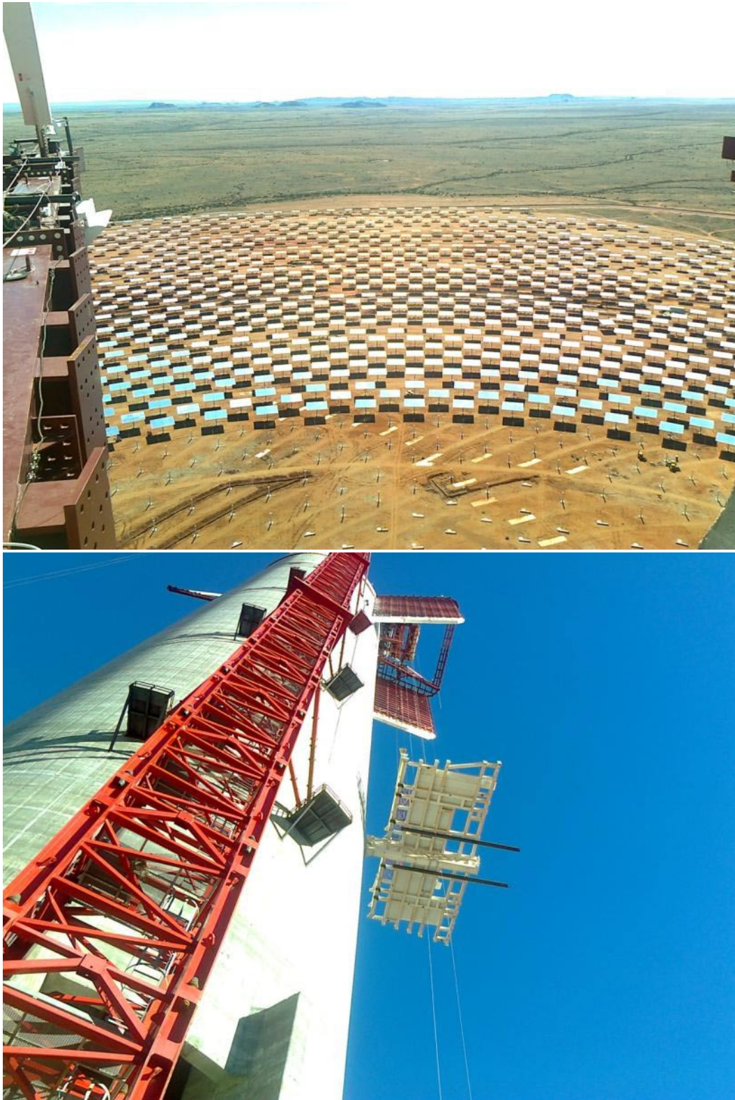
Figure 3.10. Solar field view and erection process of the Solar Receiver. Khi Solar One. Image: IMASA.
