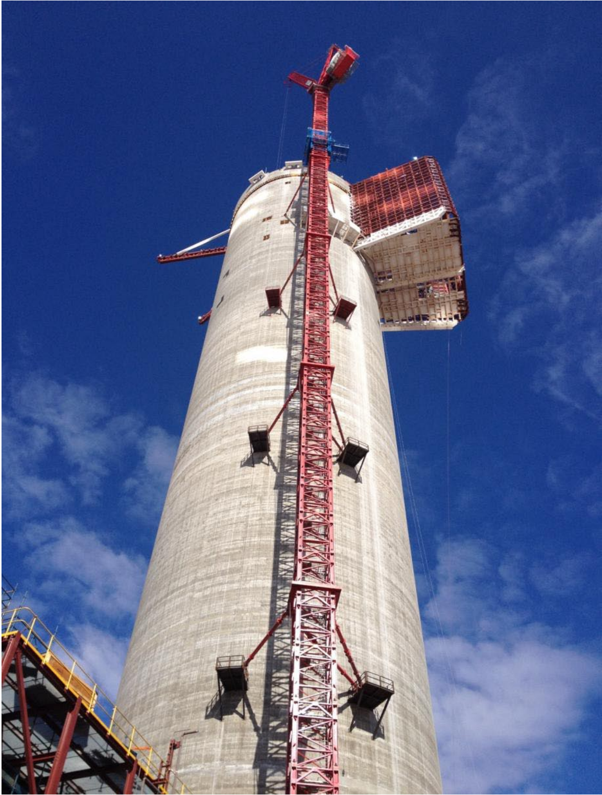
Figure 3.11. Khi Solar One Tower. Image: IMASA.
