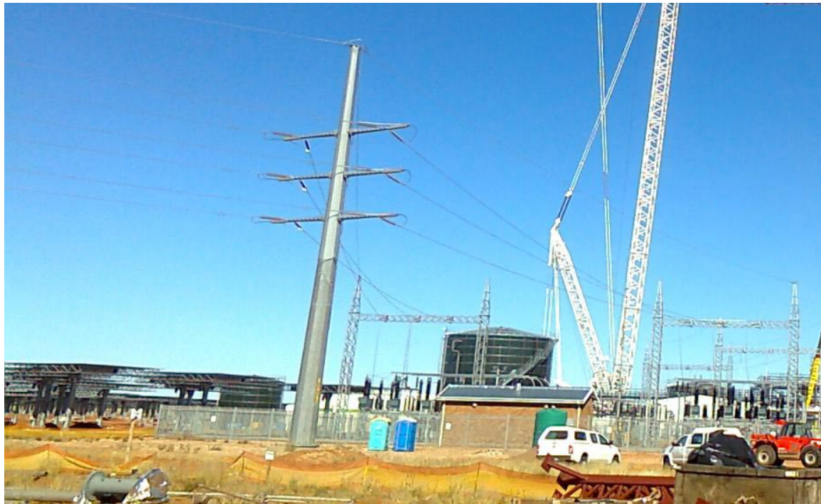
Figure 3.9. Single pole overhead interconnection between Khi Solar One and Eskom Grid. Image: IMASA.
