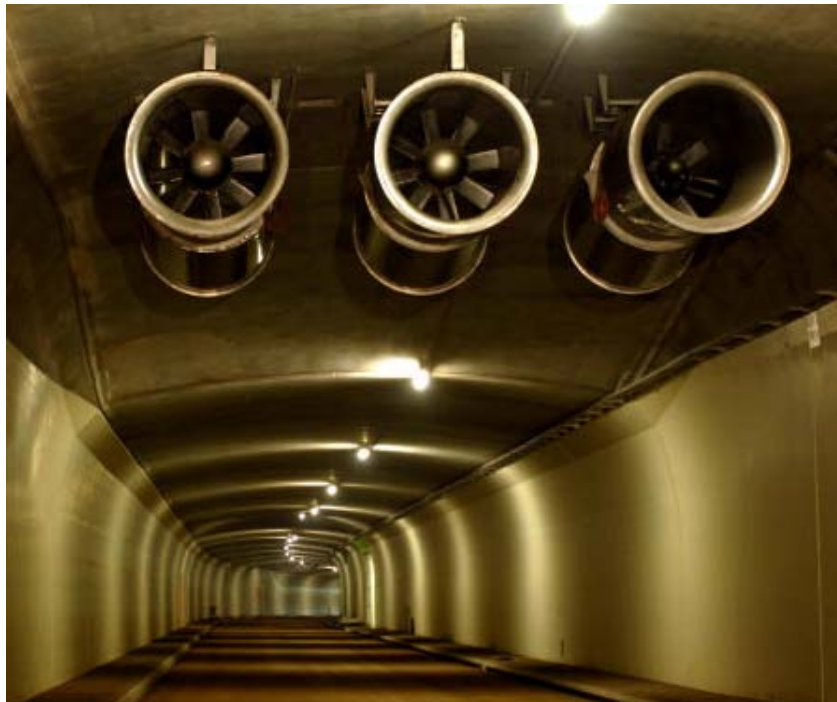
Figure 1.3: Jet fans in a tunnel
