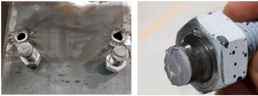
Fig. 10. Failure modes. Example of punching shear of frontal face at the studs-row in tension for joint SMS1 (left) and failure mode of the studs-row subjected to tension in joint SMS5 (right).
