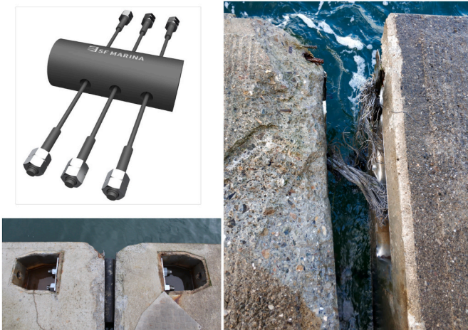
Fig. 2. Semi-rigid floating breakwater connector type (Marina) (upper left), connection installed and working properly (lower left) and broken connection after sea storms (right).
