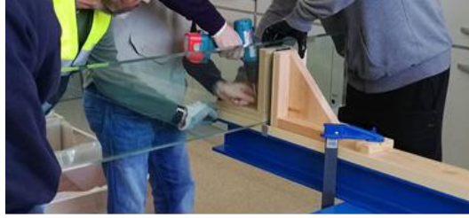
Figure 3. Fastening of the wooden lateral restraints after the placement of the laminated glass beams.
